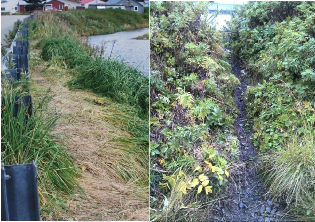
Photo 2-2. Left: Trampled Vegetation along Guardrail; Right: Noted Erosion on Upper Riverbank due to Surface Drainage
