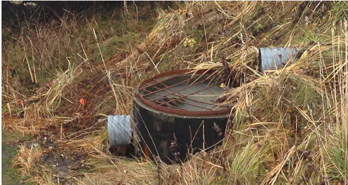
Photo 3-3. Outfall Sediment Collection System near 5th St. Bridge
