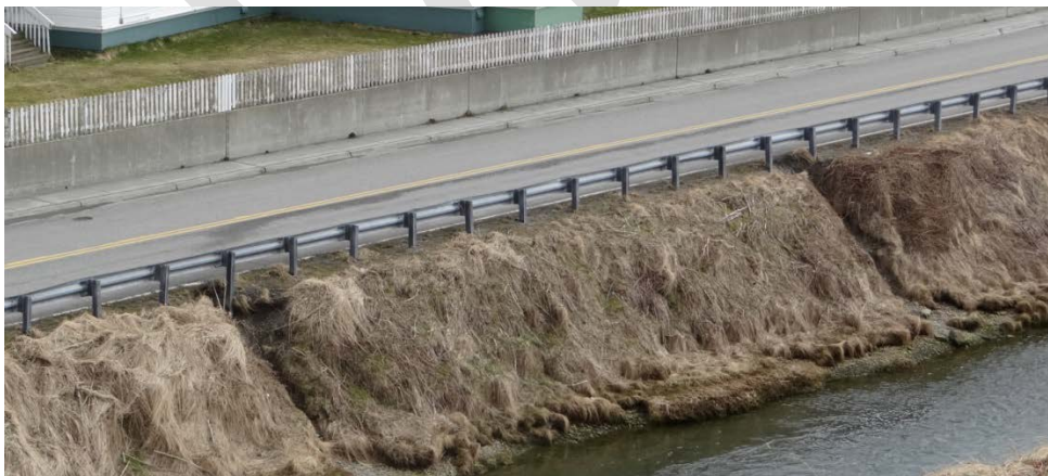
Photo 3-2. Erosion from Runoff Threatening Roadway
