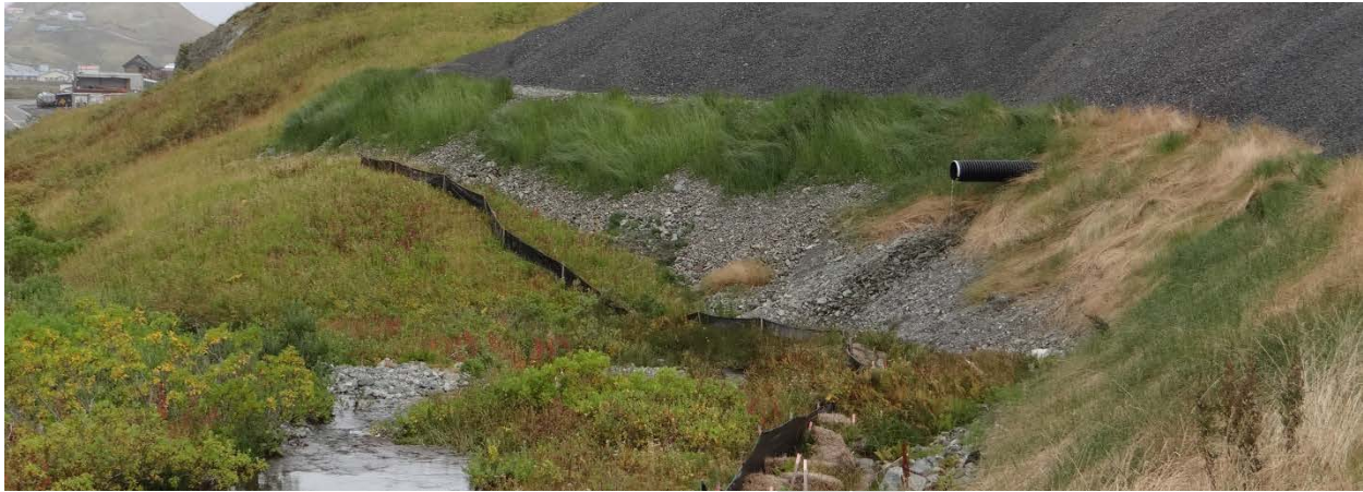
Photo 6-1. Silt Fence, Straw Wattles, and Seeded Slopes in Use at City Stockpile
