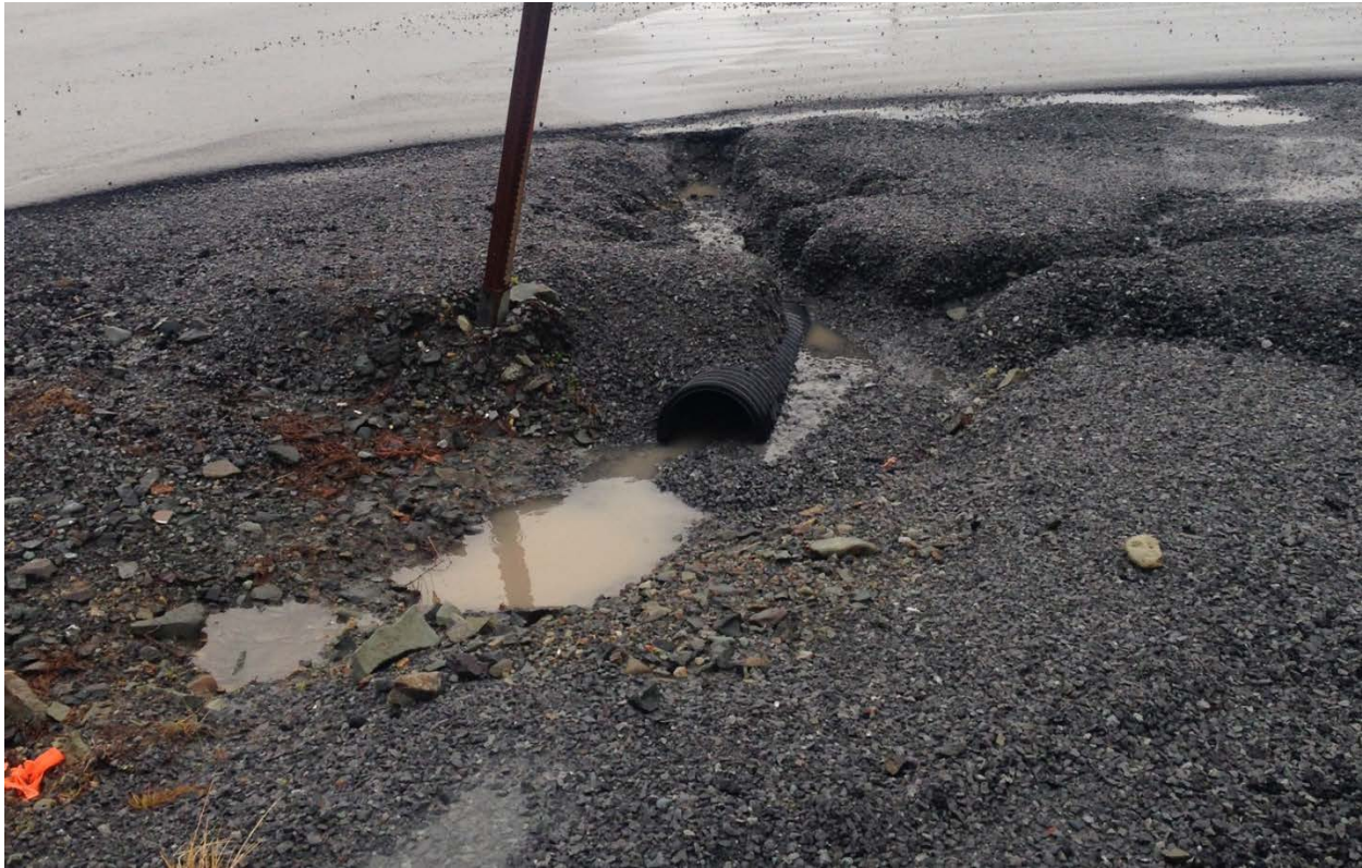
Photo 8-10. King Street/E. Broadway Intersection Culvert and Noted Erosion
