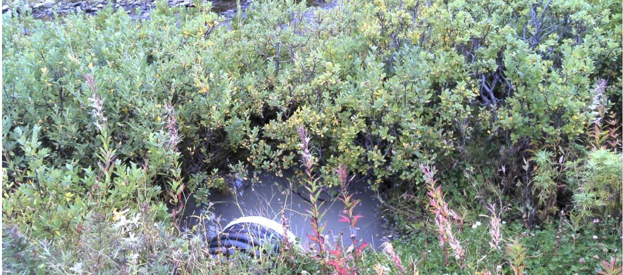
Photo 8-2. Sediment-Laden Stormwater Discharge
